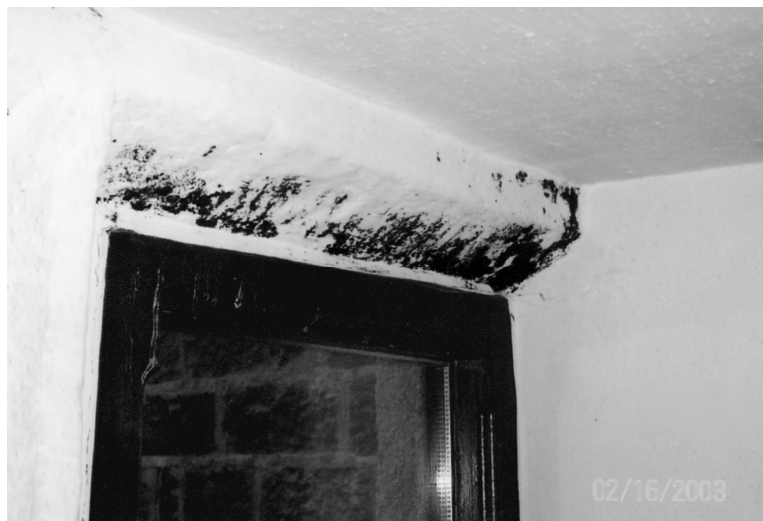
Dampness and mould staining due to a combination of surface condensation and thermal bridging in an under-heated dwelling. (Picture courtesy of Energy Inform)
