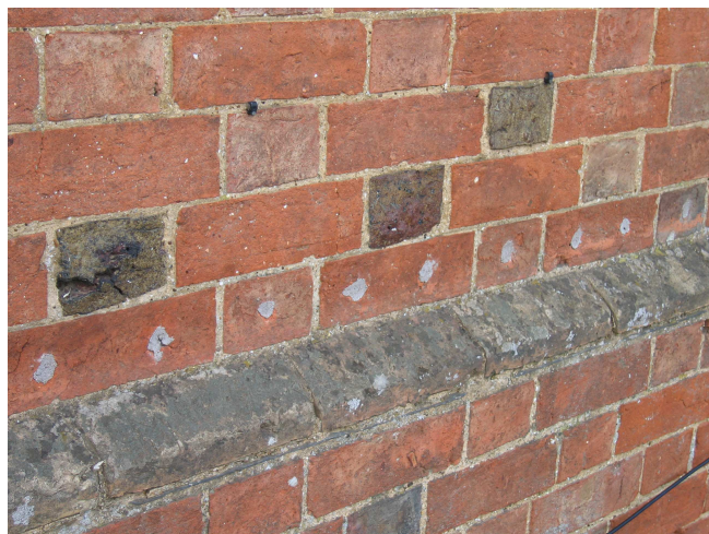
A brick wall that has had an injected damp proof course installed
