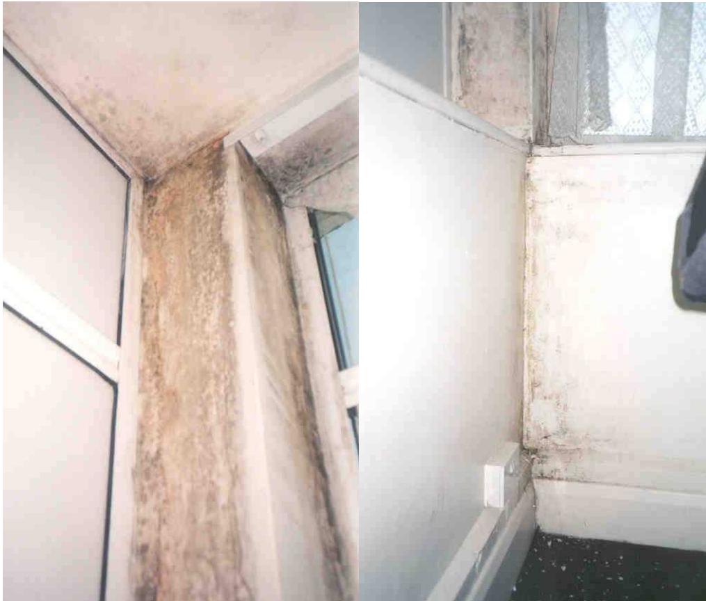
Dampness and mould staining due to condensation arising from thermal bridging in a building where the structural concrete frame bridges the wall insulation
